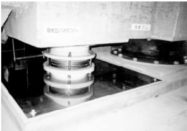
Figure 8. Photo of the friction damper with the coned disc springs in the actual base-isolation building
